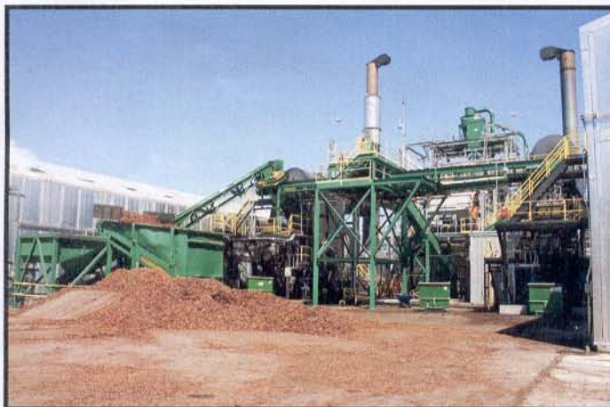
Continuous dry kilns utilize bark through a hog, metering bin and two burners.
